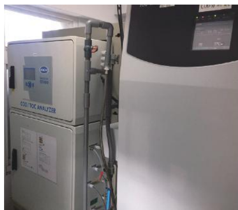
Automatic Effluent Monitoring System
